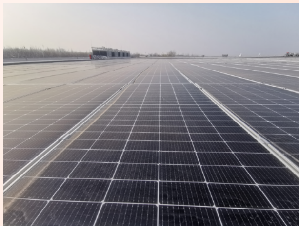
Photovoltaic Power Generation Project in Miyun
